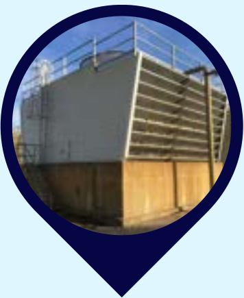
WOODEN COOLING TOWER
